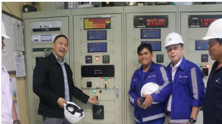
A ceremonial switching is done after the ribbon cutting ceremony with the Substation Electrical Equipment Dept. Supervisor , Engr. Richard Bulaon. (3 rd from right.)
